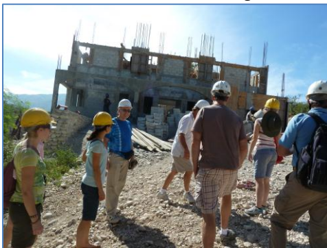
We toured the Health Center in progress. No, it is not crooked, the photographer is.
